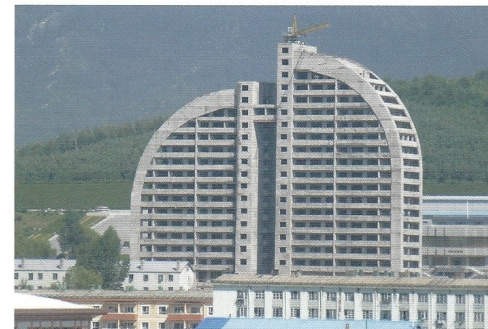
In the past years, building activities in Rason have been brisk. While official statistics are lacking, it seems to indicate also a sizeable increase of population in the area.
